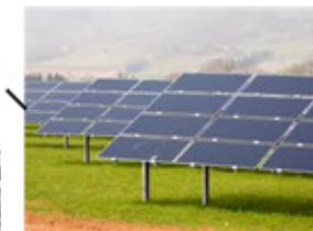
Asset #2 Solar Energy
